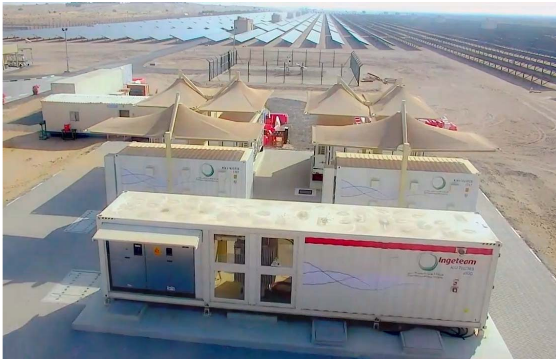
Ingeteam's power station equipped with two storage inverters and all the MV equipment.
